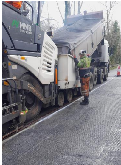
REMEDIAL WORKS ON N65 AT KILMEEN TO ADDRESS LOCALISED DEPRESSION CAUSING ROAD SAFETY CONCERN
