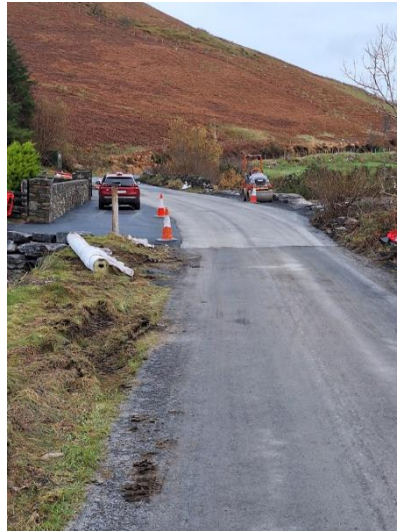
L1301 GRIGGINS- STORM BERT DAMAGE BEFORE AND AFTER
