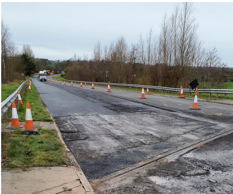
OVERLAY WORKS BEGINNING ON THE FORMER NATIONAL ROAD DEPARTMENT OF TRANSPORT GRANT FUNDING R446 AUGHRIM TO BALLINASLOE AT URRAGHRY
