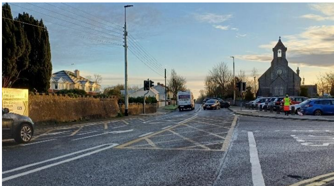
UPGRADE WORKS ONGOING TO IMPROVE PEDESTRIAN CROSSING FACILITIES AT SHANNONBRIDGE ROAD AND OLD DUBLIN ROAD LEGS AT CREAGH JUNCTION, BALLINASLOE
