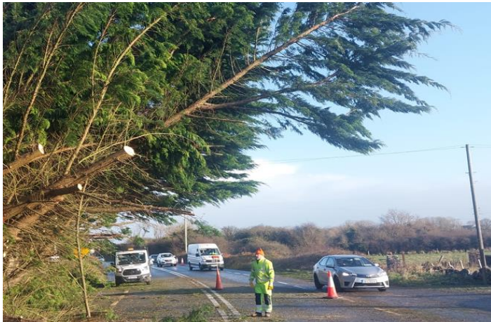
STORM CLEAN UP – N83
